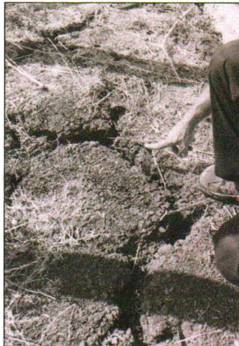
Figure 2: This crack is at least 32 inches deep. The yardstick was easily inserted to this depth; narrower, less straight cracks may extend much deeper.
